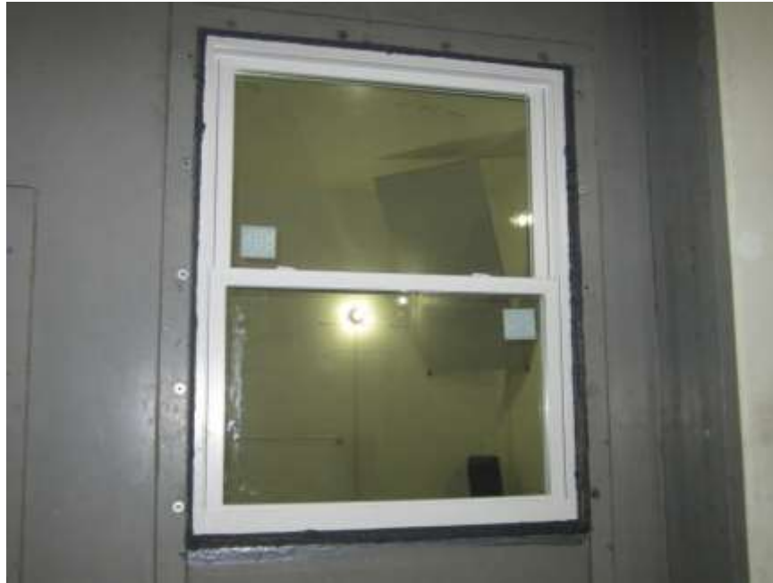
Receive Room View of Specimen Installation
